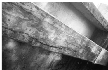
Cracking parallel to bars
