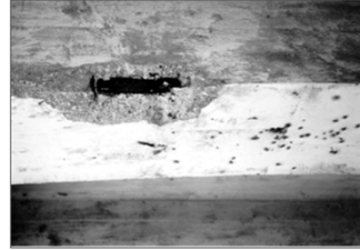
Exposure of bar in a beam angle due to corrosion
