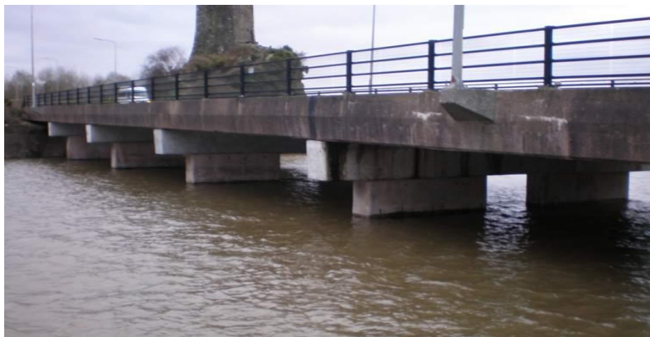
Fig. 20. Photograph of effects of failed expansion joint
